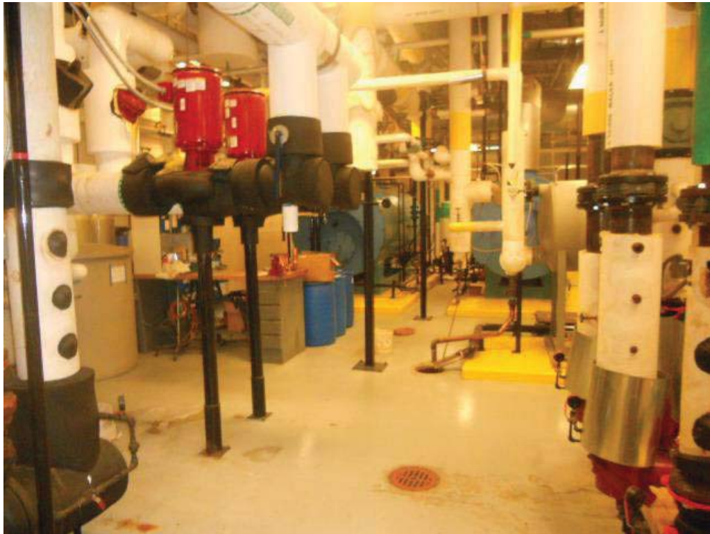
Basement Level - Boilers
